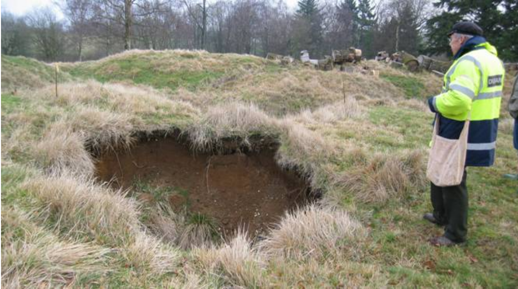
Figure 4: Ground subsidence resulting from failure of a dugout at the Beaumont Hamel Memorial Site. The parallel ridges, running across the photograph from left to right, mark the top of the trench line. This subsidence event is located in the part of the site which is fenced to prevent public access.
