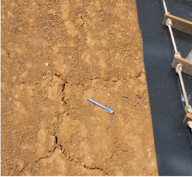
Figure 2 Desiccation cracking of CCL before the GM is placed
