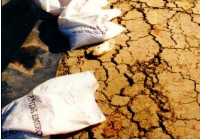
Figure 3 Compacted clay liner (forming part of a composite liner) that has desiccated (Photo courtesy of P. Davies).
