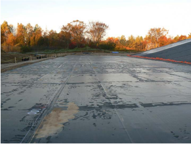
Figure 8 Photo of a GM in direct contact with the underlying GCL liner at QUELTS at 7:00am on a cool October morning. Note: right-left distance from toe of slope to anchor trench is about 20m.
