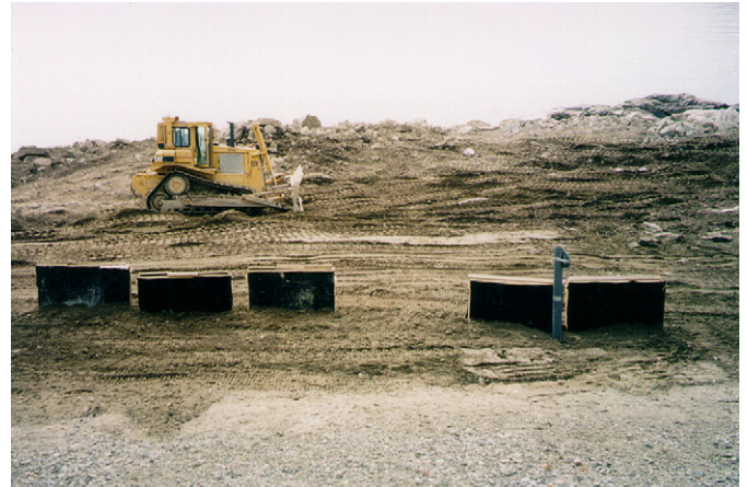
Fig. 1. Photograph of frames supporting f-HDPE GM coupons during installation and prior to complete soil burial and placement of GM surface cover.
