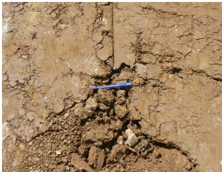
Figure 5. Photograph of a poor surface of a clay liner.
