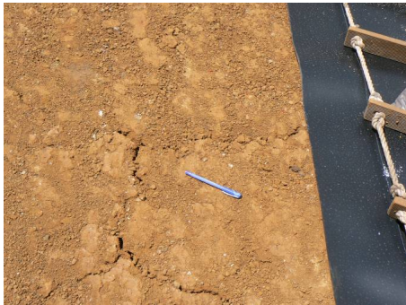
Figure 4. Photograph of a clay liner just before placement of overlying GM. Note desiccation cracks.
