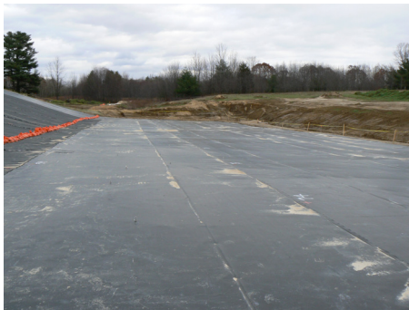
Figure 1. GM with essentially no wrinkles (in direct contact with the underlying clay liner); cloudy early November morning when ambient temperature 3°C.
