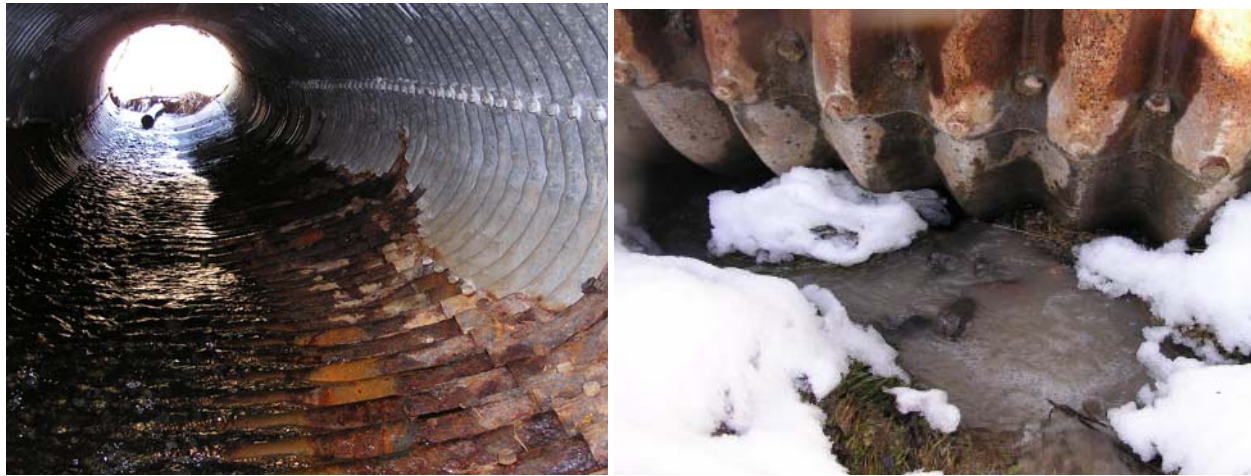
a. Invert corrosion.
