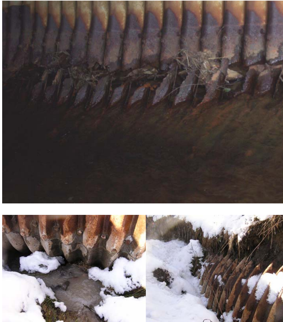
Figure 1. Erosion takes place due to water percolation through corroded zones (culvert in South Eastern Ontario).
