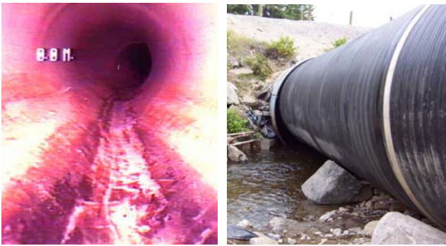
a. Clay sewer after repair b. Slip-lining of corroded metal culvert in Northern Ontario. Figure 8. Damaged pipe repair using liners
