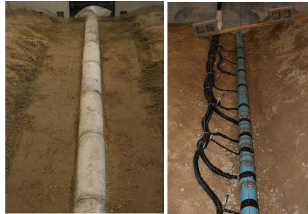
c. Concrete sewer d. Adjacent PVC water pipe Figure 16. Pipe bursting test, Cholewa et al. (2008).
