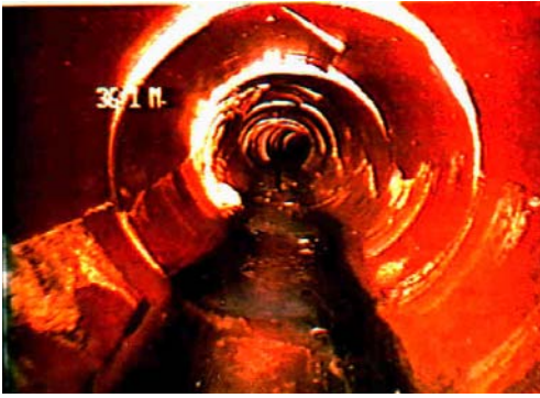
a. Fractured Clay Sewer in Toronto.
