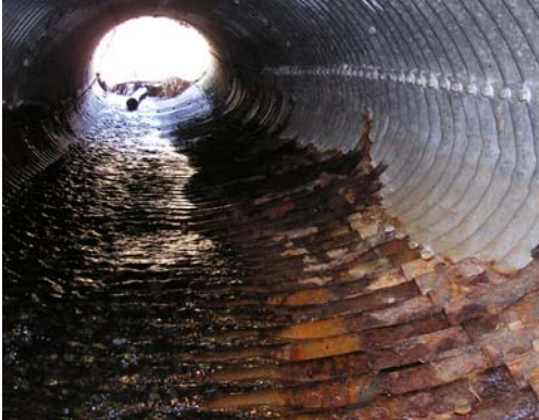
b. Corroded metal culvert in Eastern Ontario
