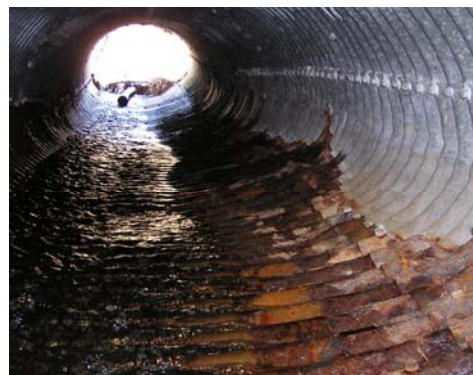
b. Corroded metal culvert in Eastern Ontario
