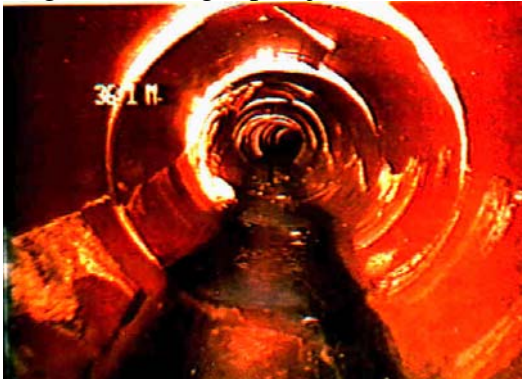
a. Fractured Clay Sewer in Toronto.
