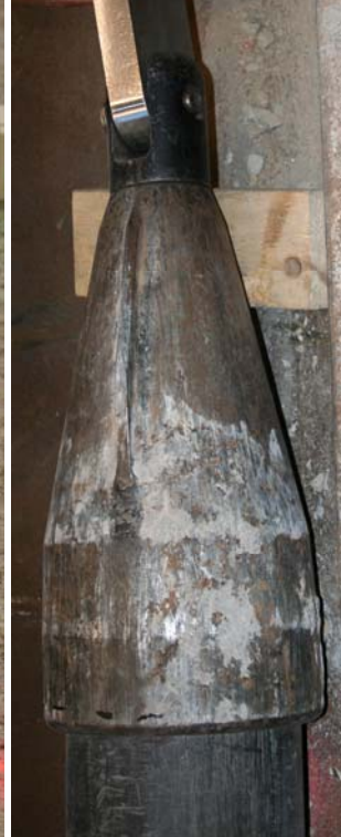
f. Burst head & new pipe
