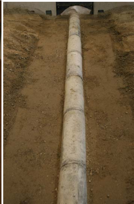
b Concrete pipe to be replaced
