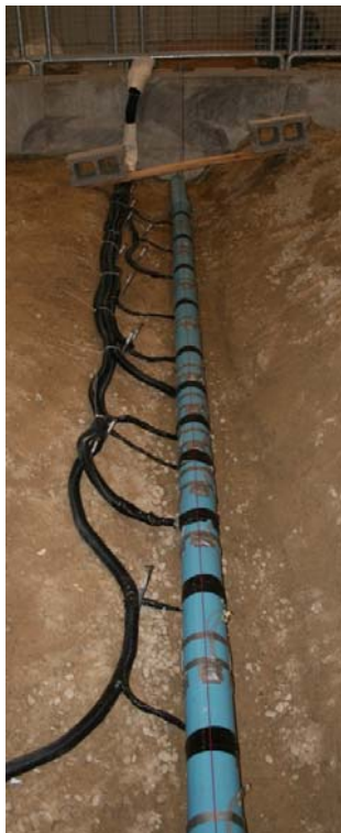
c. PVC pipe with gages.
