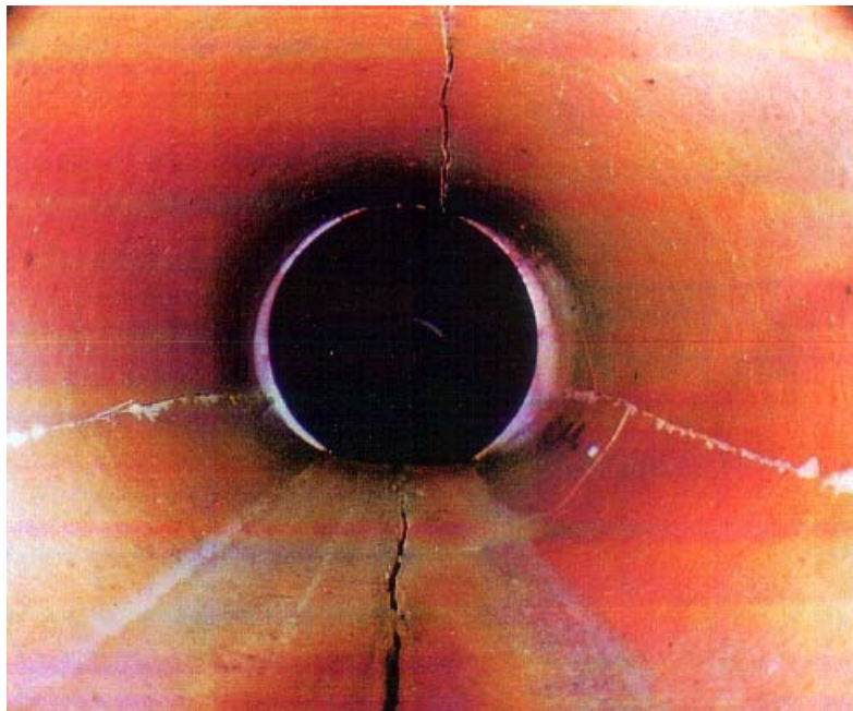
Figure 1 – Rigid Pipe with Overloading Fractures (with permission, [5])
