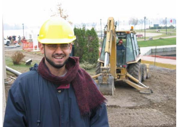
Abdul inspecting a pipeline rehabilitation project in Gananoque, Ontario, an excursion organized by the Queen's University Student Chapter of NASTT, 2006.
